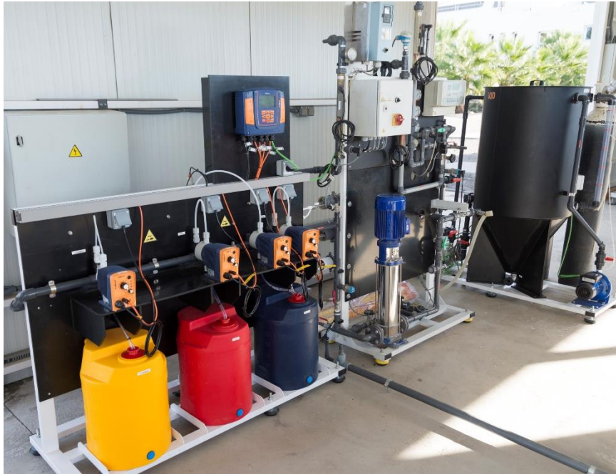
Figure III.12: The pilot plant for NF available at the PSA
